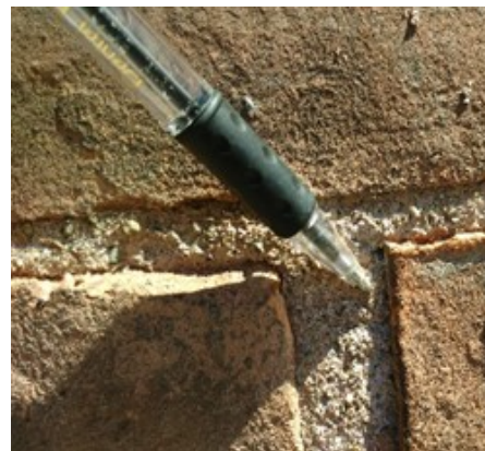
Soft mortar will shed granules of sand when scratched with a key or a pen.
