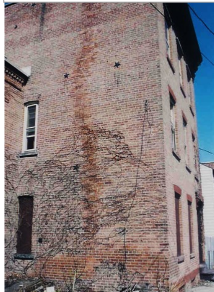
This damage traces the length of a chimney. The temperature differential has eroded the masonry. Repointing is useless without lining the chimney first.
