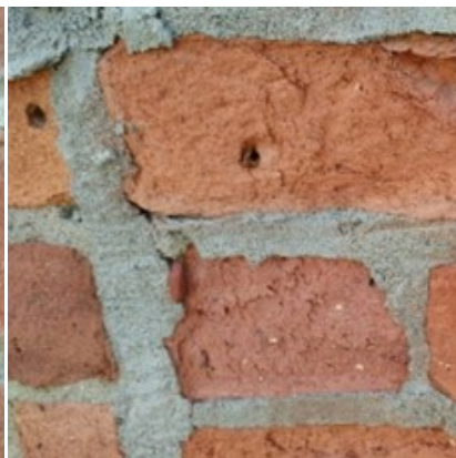
The use of hard mortar has caused the face of these bricks to spall.
