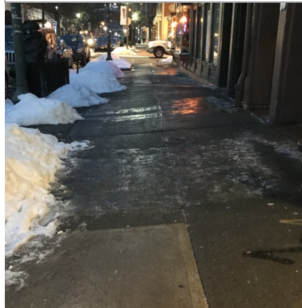
Don't allow building drainage to drip on a sidewalk and create dangerous icing.
