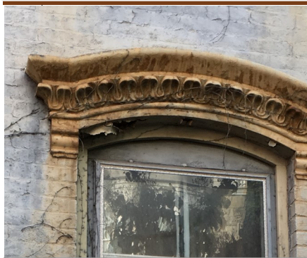
Proper preparation and paint will ensure the longevity of this metal window hood, masonry wall and wood windows.
