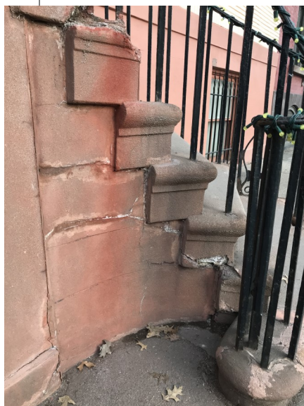
It is best to determine the reason for the damage and to eliminate that threat to the stone before making repairs.
