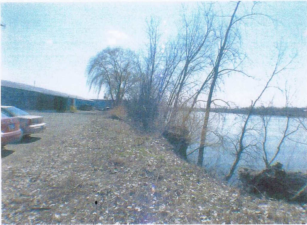
15. View south from the Bruno Machinery property. The trail will extend along the top of the embankment.
