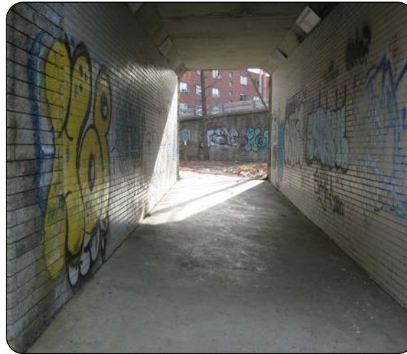
Photo 4: Graffiti painted pedestrian tunnel under bridge ramp.
