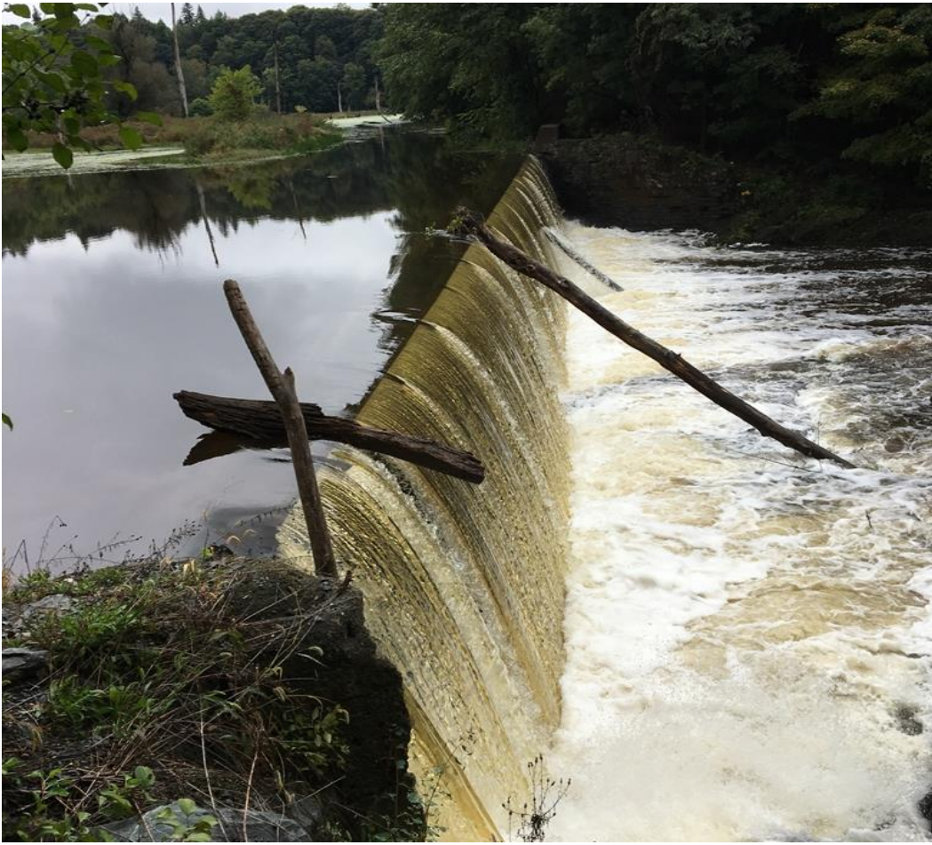
Photo 1 Dam ID# 226-1391 Ida Lake Dam 09/28/2018 Dam crest looking toward the left abutment
